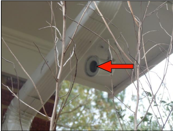
Front right corner floodlight
