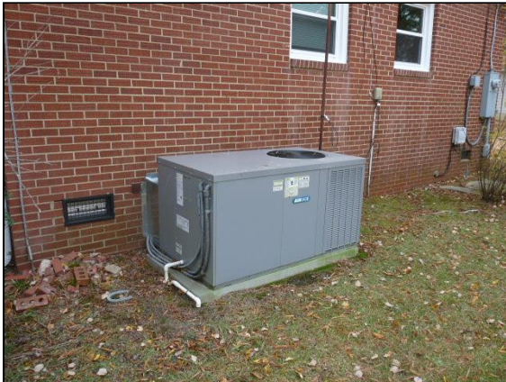
HVAC package unit on the right side of the house
