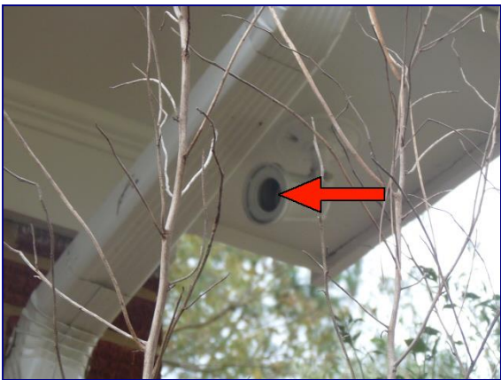
Front right corner floodlight
